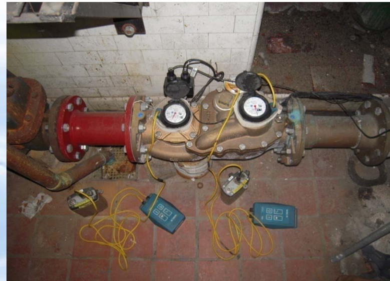
Data-logging consumption on a 4-inch compound meter in an urban high school
