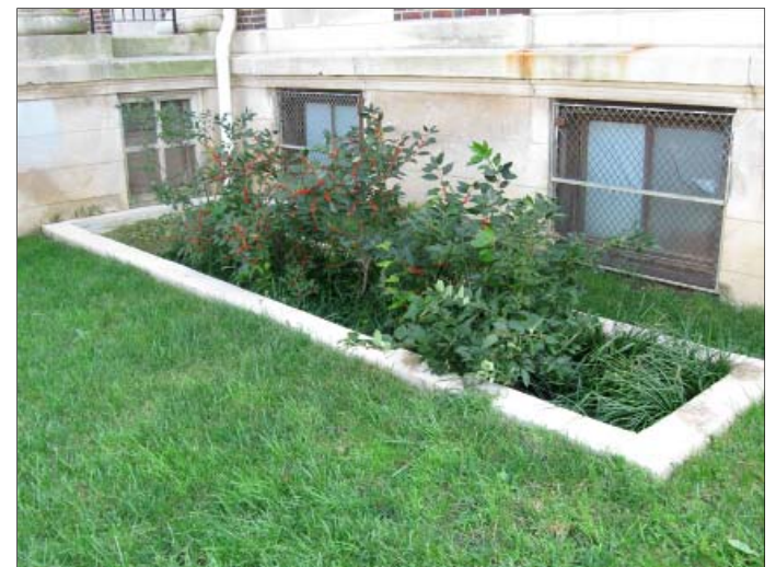
Downspout Planter: Waterview Recreation Center Germantown
