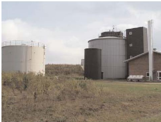
Large Scale Centralised Co-digestion Plant Grindsted, Denmark (Picture courtesy of Rudolf Braun, Austria)
