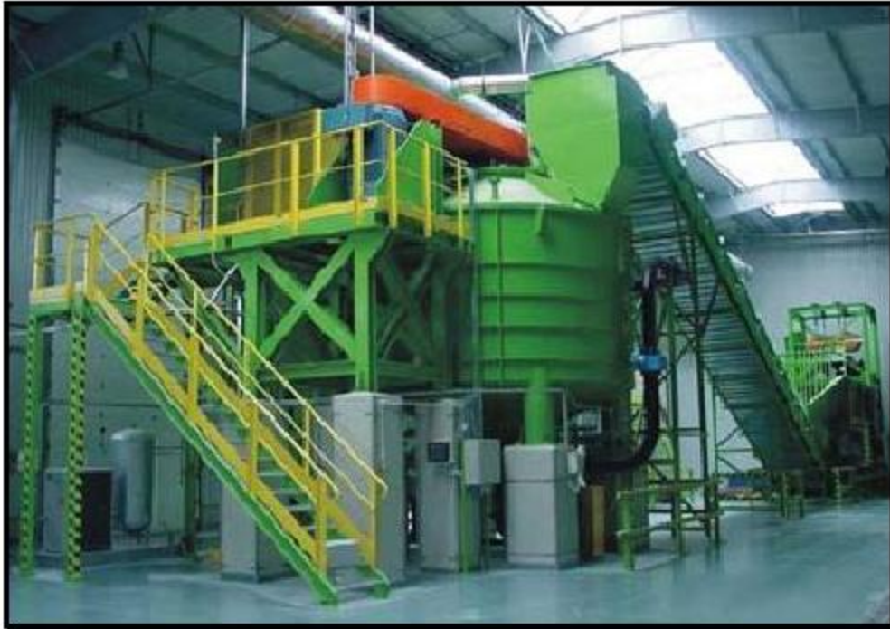
Hydropulper & Grit Removal System
