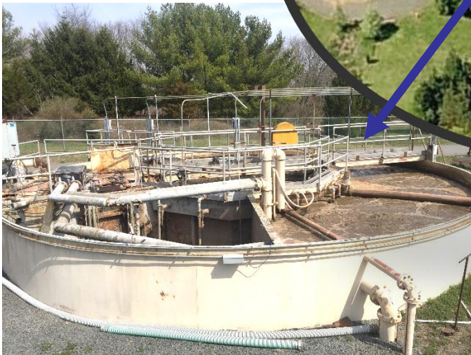
Equalization/ Clarifier Tank
