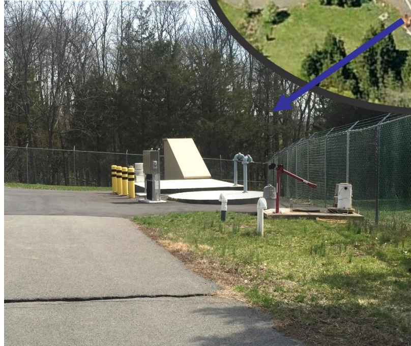
Wet Well & Dry Well
