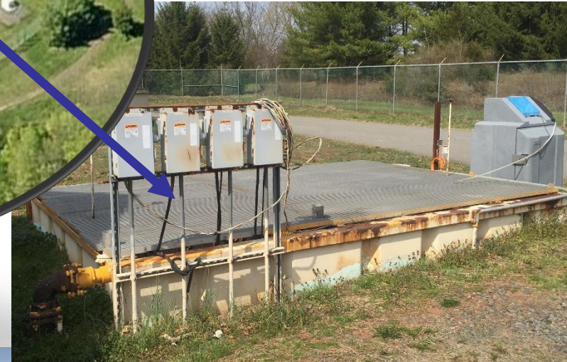
Post Aeration Tank
